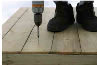
Step 14 - The shed roof is screwed down into the top of the side panel framework from the outside.
