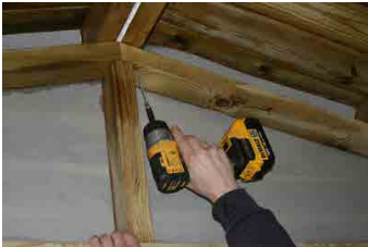
Step 13 - All side panel framework can be screwed up into the roof panel framework.
