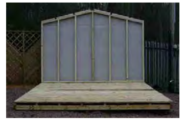
Step 4 - With the floor in place, each panel can now be positioned & screwed together starting with the back panel.
