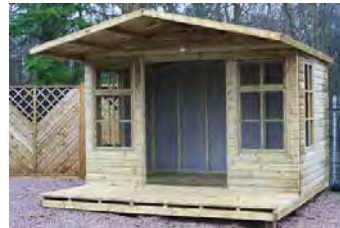
Step 11 - The first roof section is put in place. Then fit the second side. Ensure butted tight to back panel.
