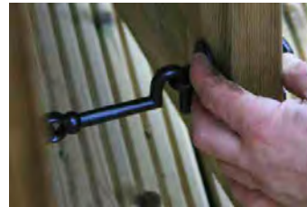
Step 33 - A cabin hook has been supplied for each door - fix to solid part of front, ensuring position will reach door without strain.
