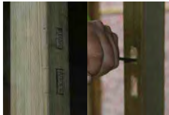
Step 32 - Mark out on LH door where the lock will fit into the door when closed. Cut out the marked area using a chisel and fit keep.
