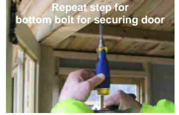
Step 30 - Mark on top of frame where a hole will need to be chiselled out in order to house the bolt & secure the door.
