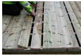
Step 3 - Loose floor boards will be provided which needs to be installed to cover the gap between the floor panels.
