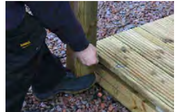
Step 16 - First, ensure the roof overhang is running level then position the support posts and mark with a pencil how much post needs to be removed.
