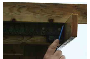
Step 26 - The side edging boards are then cut to fit and nailed to sandwich the felt along the roof edge.
