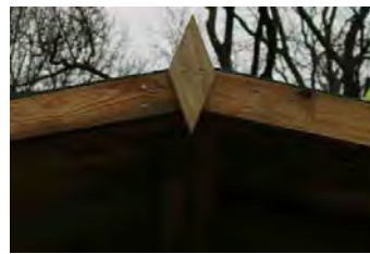
Step 25 - Roof front and rear panel edging boards are cut in the center and nailed to sandwich the felt + nail on diamond in center.
